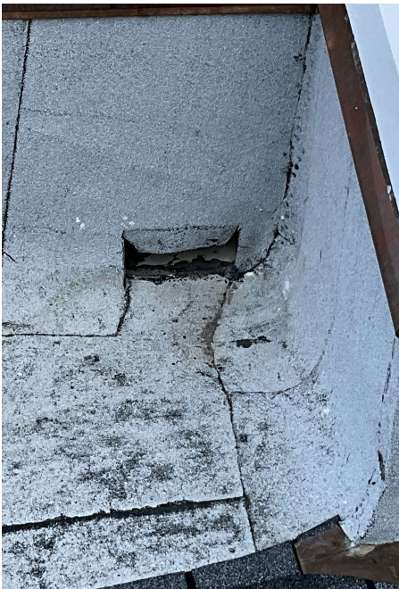
4 Scuttle hole to be repaired.
